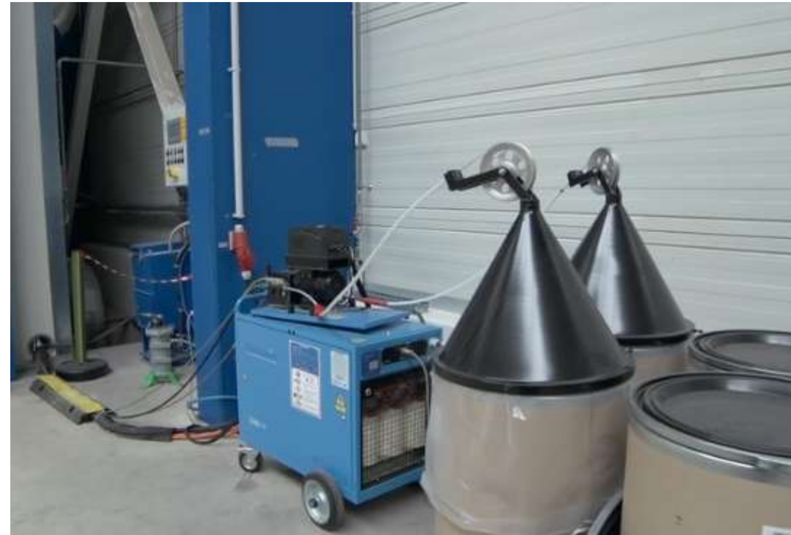
Zinc fill station
