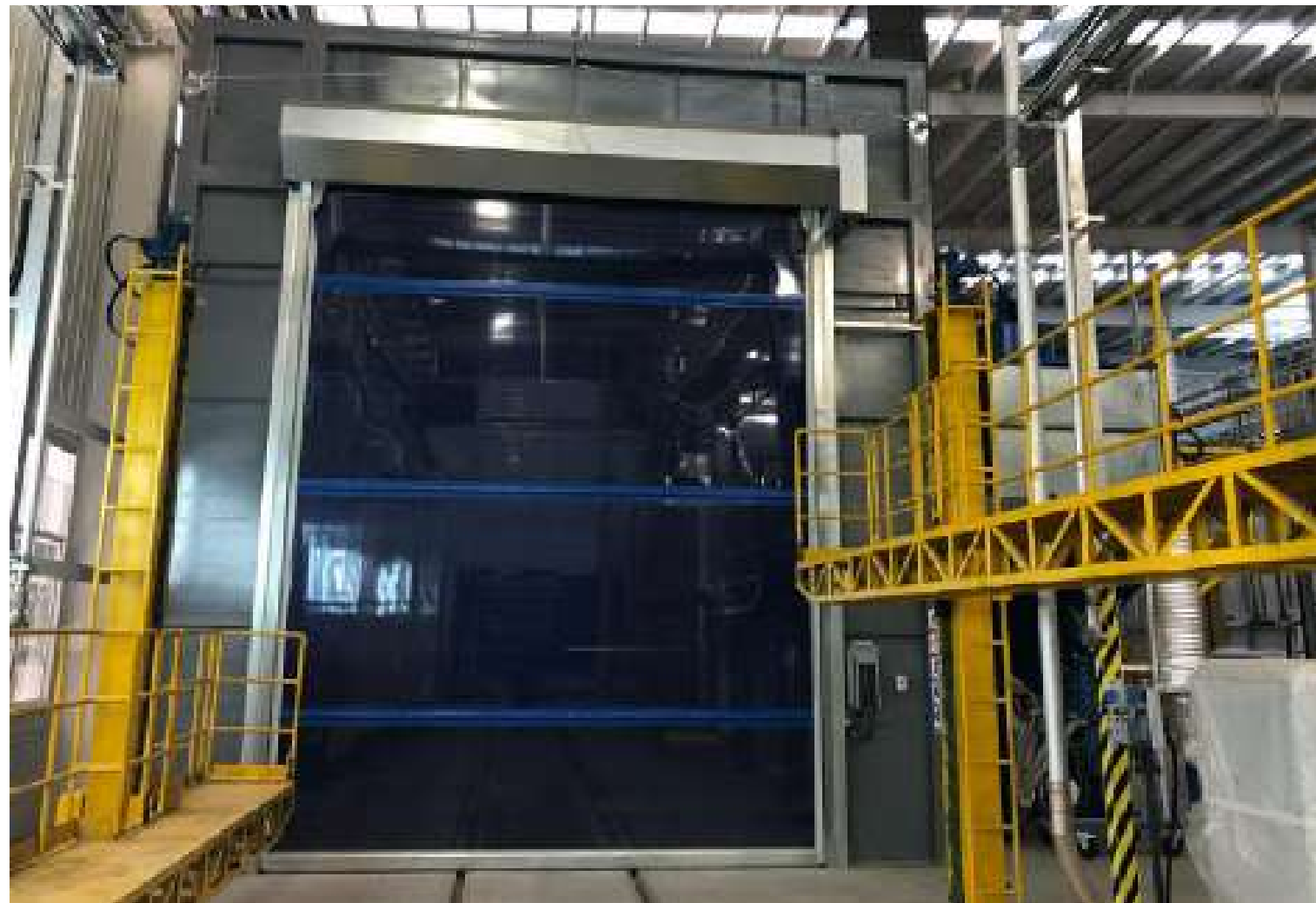
Sandblasting room with two electrically operated roller doors on the frontal sides
