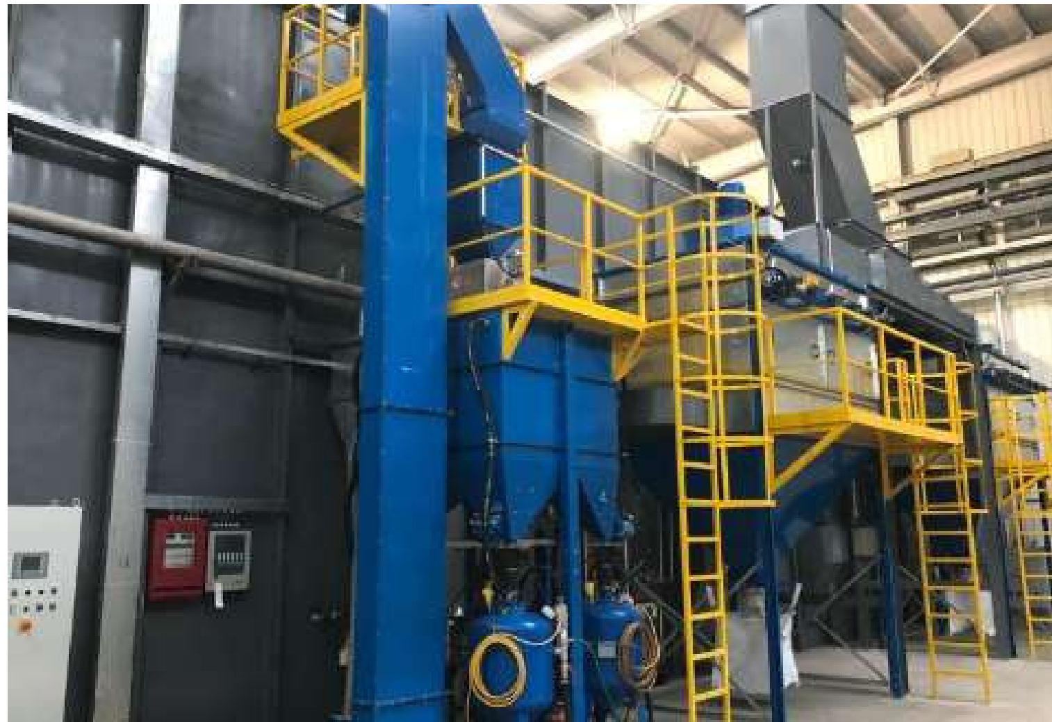
Abrasive silo and filter plants with maintenance platforms
