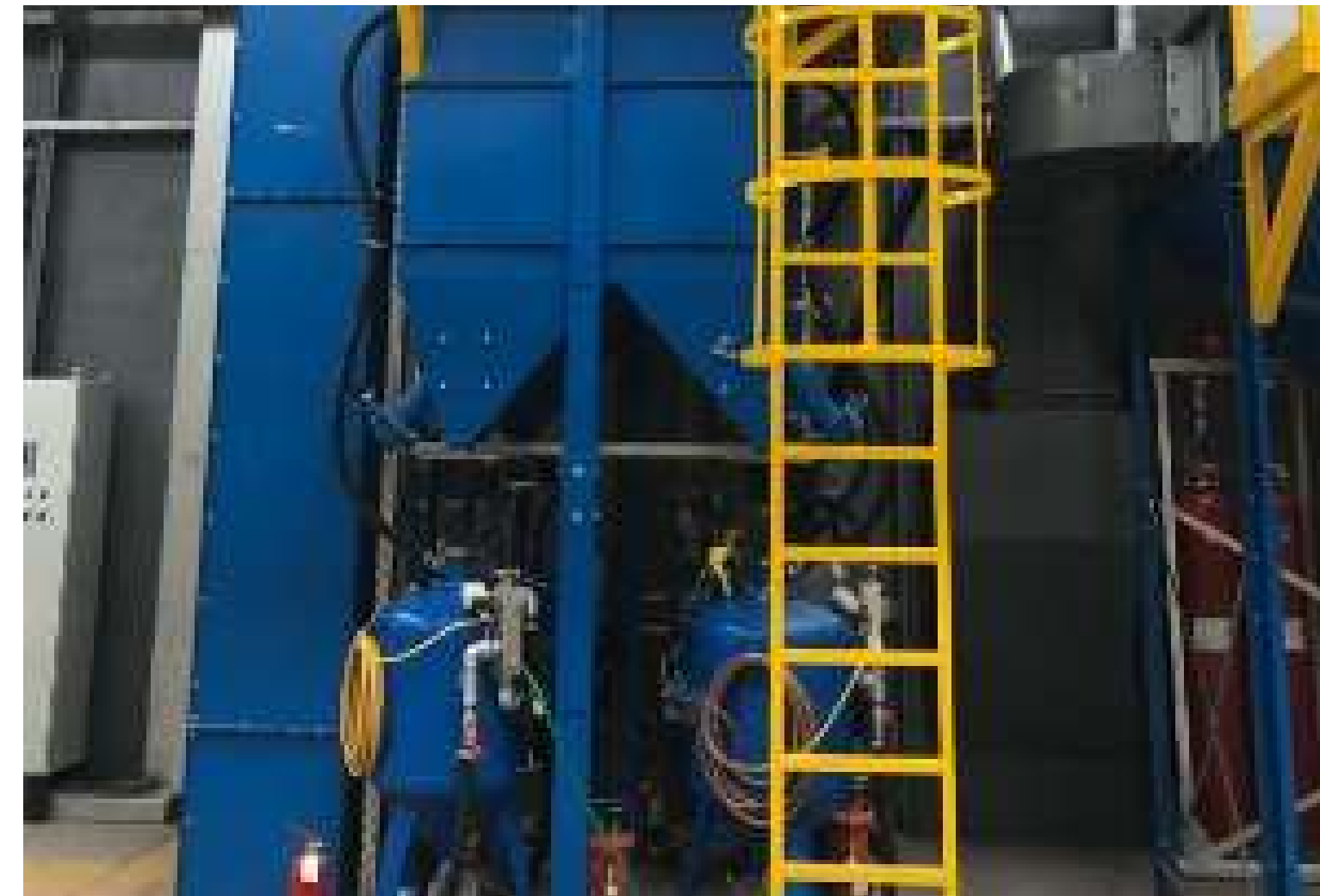
Abrasive silo with four pressure sandblasters
