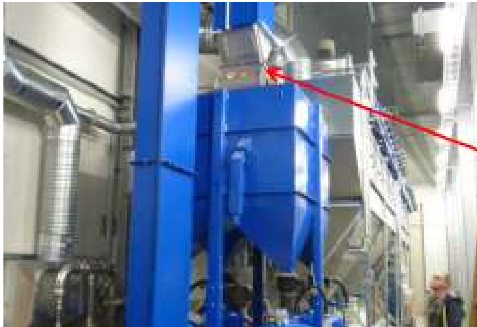
Machine room with filter unit
